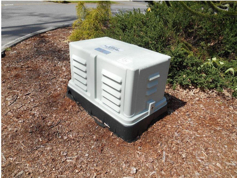
Figure 3 - Example of an Autoflush location
